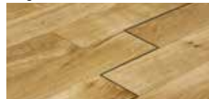
Irregular gaps formed due to edge bonding
